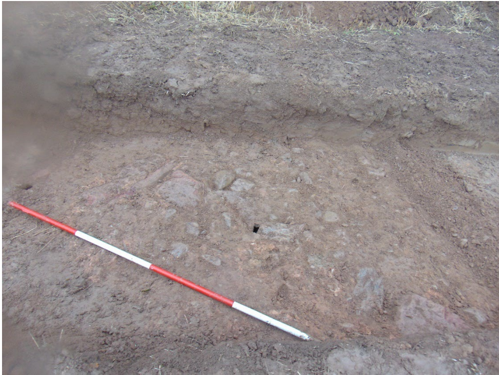
Plate 47: North facing shot of culvert. Stone drainage still in use. 2m ranging pole. Trench 1240.
